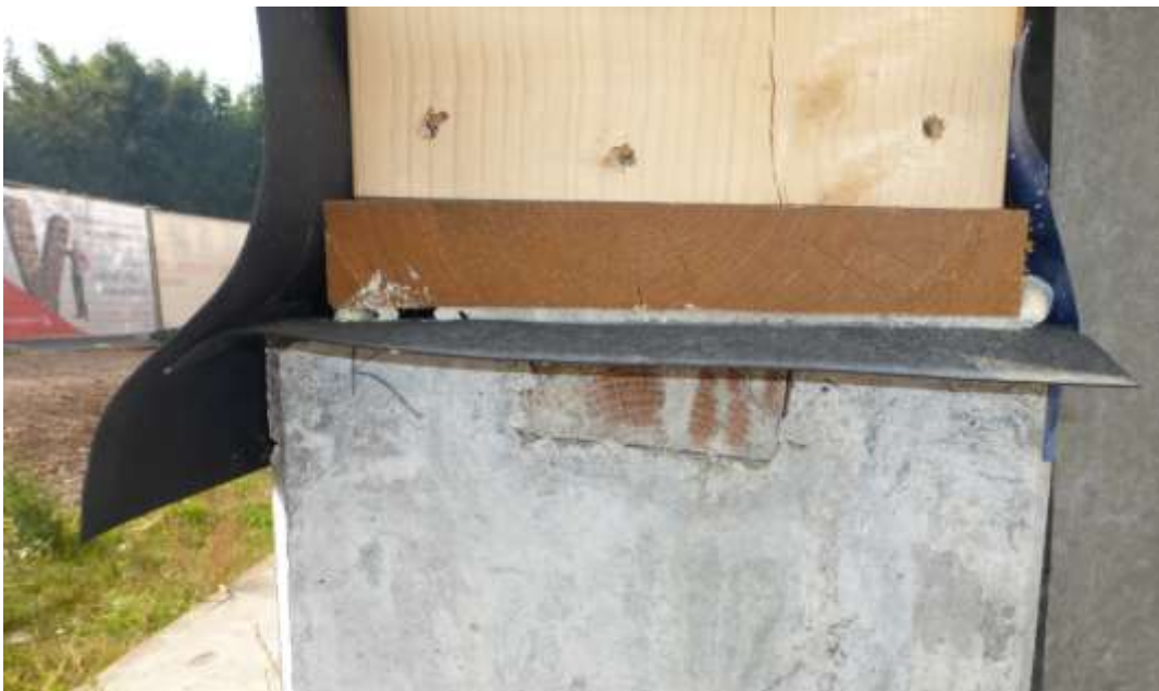
Figuur 104. Ingegoten houten regel in betonpaneel.
